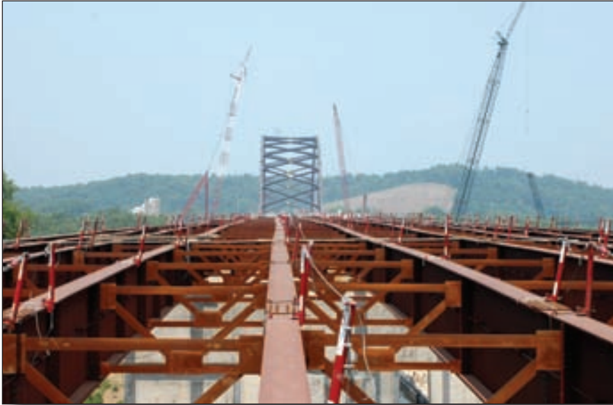
The bridge's arch span is strengthened by post-tensioned steel cables configured in an X-shaped network to enhance stiffness and redundancy in the bridge's superstructure.
