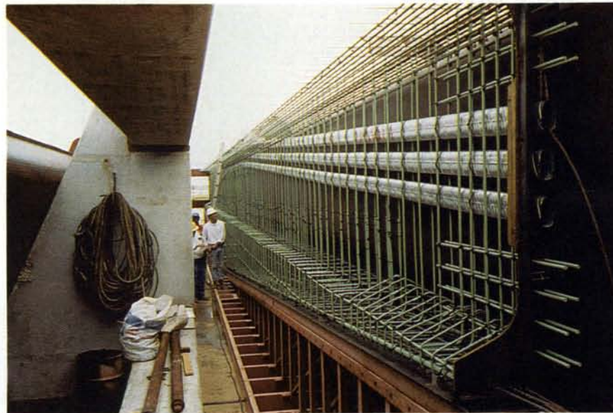
Fig. 7. Forms, post-tensioning ducts and mild steel reinforcement used in casting haunched girder section.
