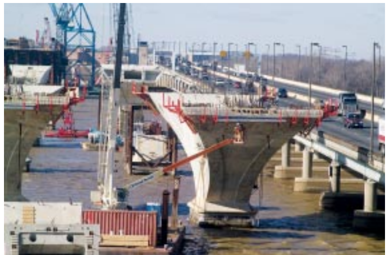
Tight Quarters. Until existing bridge (right) is demolished, it restricts amount of space available for working on new northern bridge (center).
