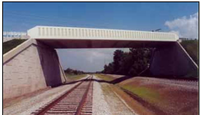
Sedley Bridge, Porter County, Indiana.
