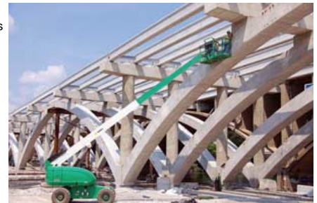
The new Fox River Bridge will be supported by 10 spans underneath the roadway, including a series of five, 178-foot-long arch spans to replicate the design of the existing bridge.
