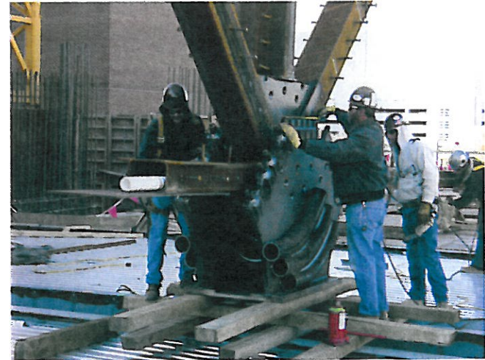
Fig. 7: HSS trusses spanning over 132 ft (40 m) formed an internal skeleton that was used to support the formwork while the concrete transfer trusses were constructed
