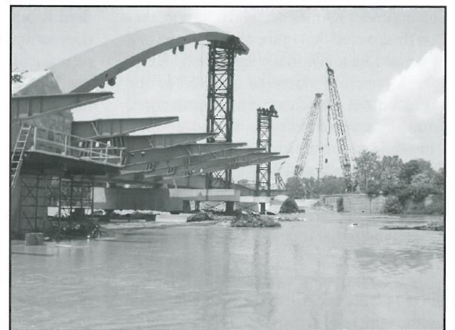
Inclined arch and bike/walkway erection underway at Main Street Bridge in Columbus, OH
