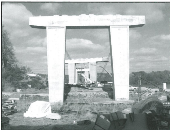
Massive concrete piers will support the new Blennerhassett concrete bridge deck and overhead arch
