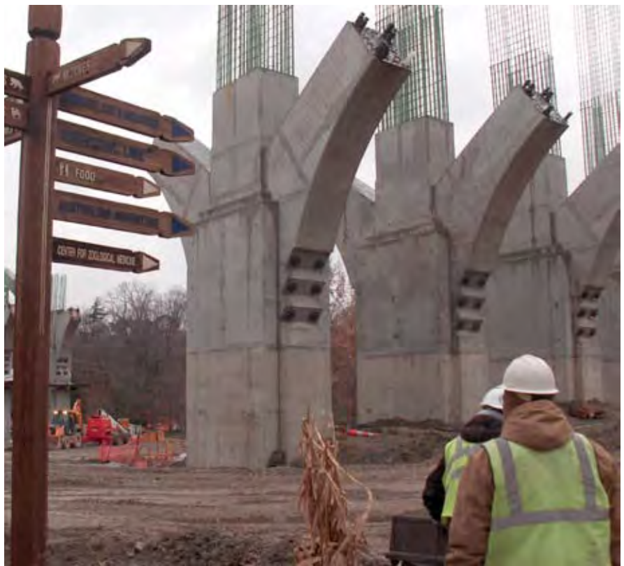
Thrust blocks located within the Cleveland Metroparks zoo. Photo: Ohio Department of Transportation.
