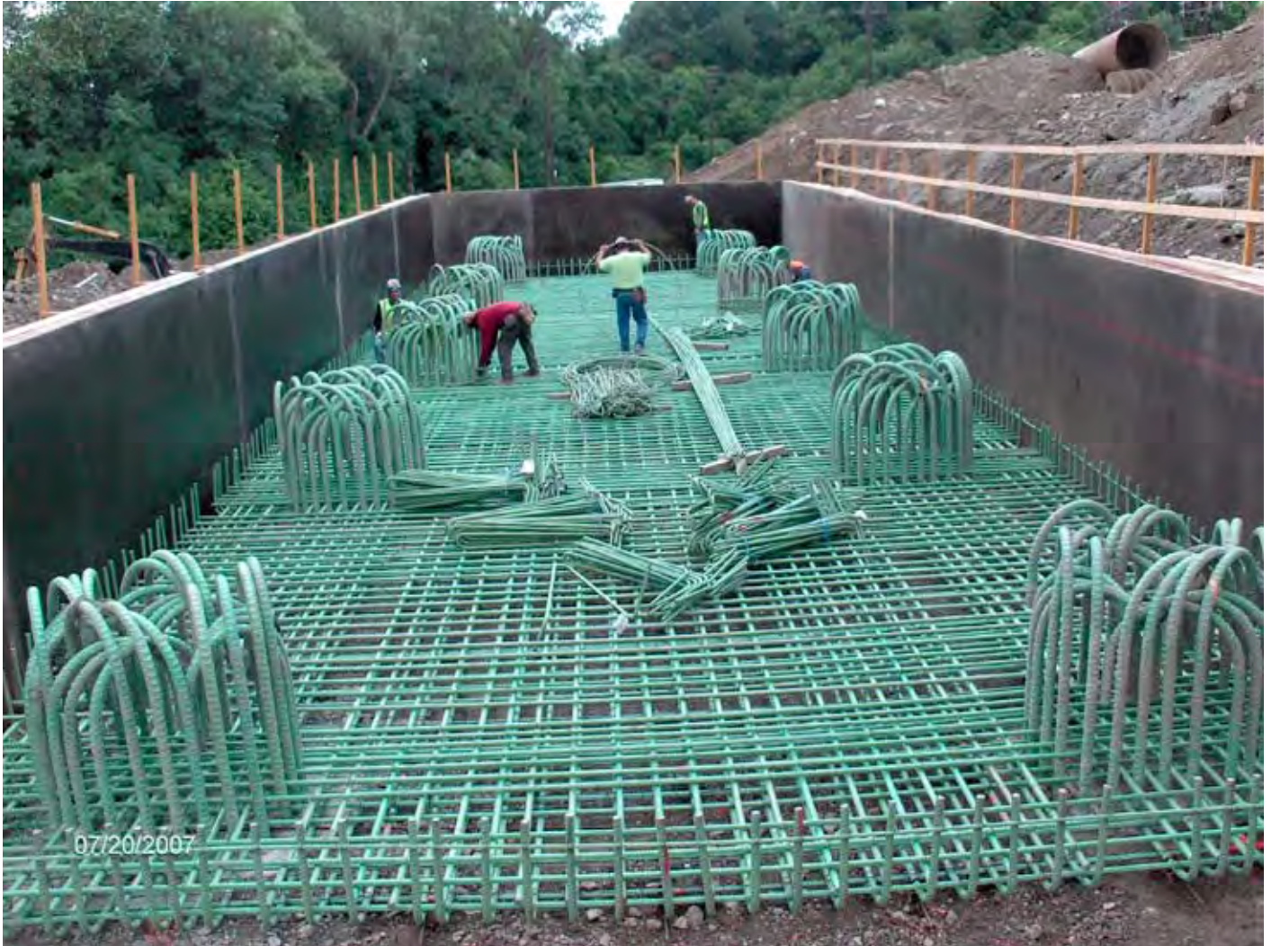
Reinforcement in the footing on 6-ft-diameter drilled shafts. Photo: Ohio Department of Transportation.
