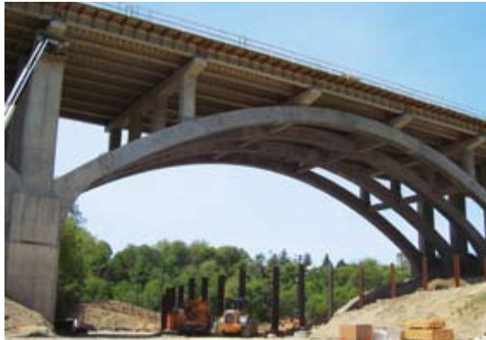
The Fulton Road bridge replacement project in Cleveland, Ohio, features 35 spans of AASHTO Type III precast concrete girders supported on five approach spans and six 210-ft-long precast concrete, post-tensioned arch spans with cast-in-place concrete piers, spandrel columns, and transverse cap beams. The bridge spans a park, the city zoo, a creek, and two active railroad lines.
