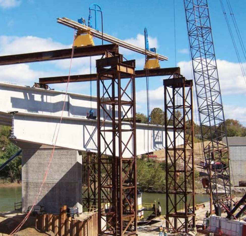
The Kentucky Route 22 project in Gratz, Ky., was redesigned by JSE from a steel-plate girder bridge to a four-span, 909-ft-long spliced bulb-tee girder design that saved about $800,000 from the previous design. The 325-ft main span provides a record length for construction of this type. Photos: Janssen & Spaans Engineering.
