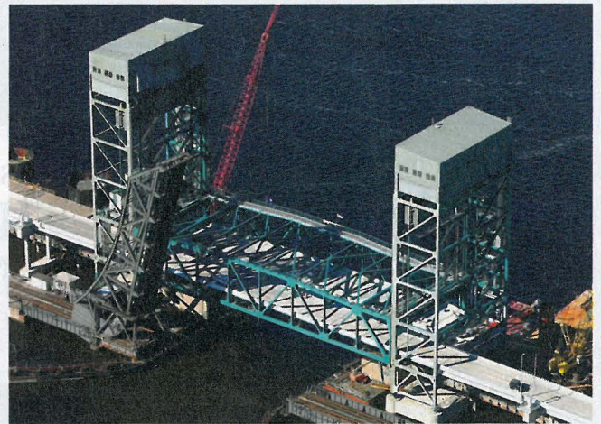
The new 1,908-ft, four-lane bridge will have a vertical clearance of 35 ft in the closed position, compared to the existing 11-ft clearance.
